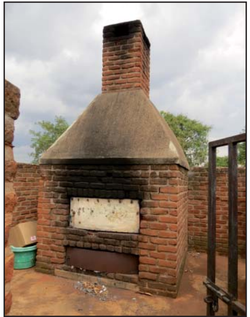
Incinerator at Machinjiri Health Centre
